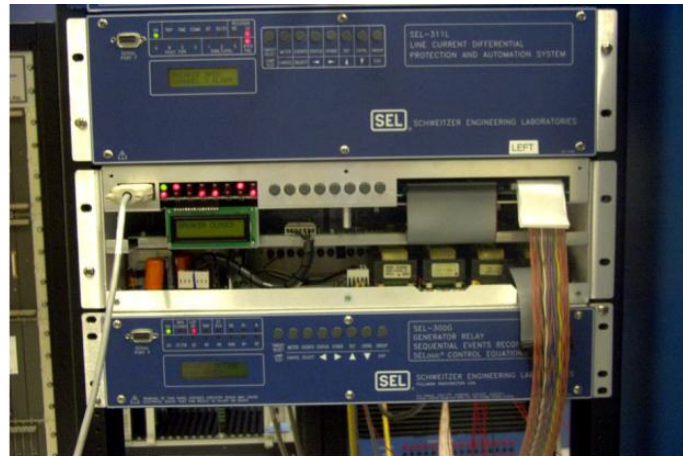
Fig. 6. Typical connections to SEL relay [9]
